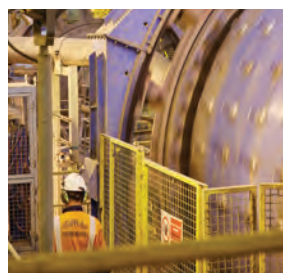
Inside the Efemçukuru processing plant, Turkey.
