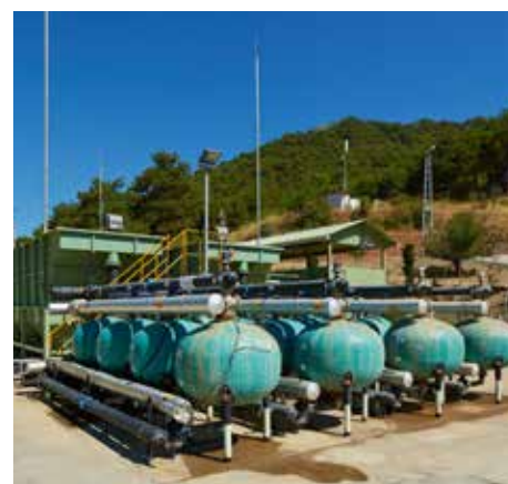
▲ Water treatment plant at Efemçukuru, Turkey.
