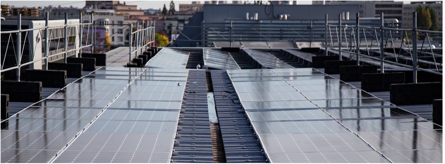
Solar panels installed at the BD European Headquarters in Eysins, Switzerland.
