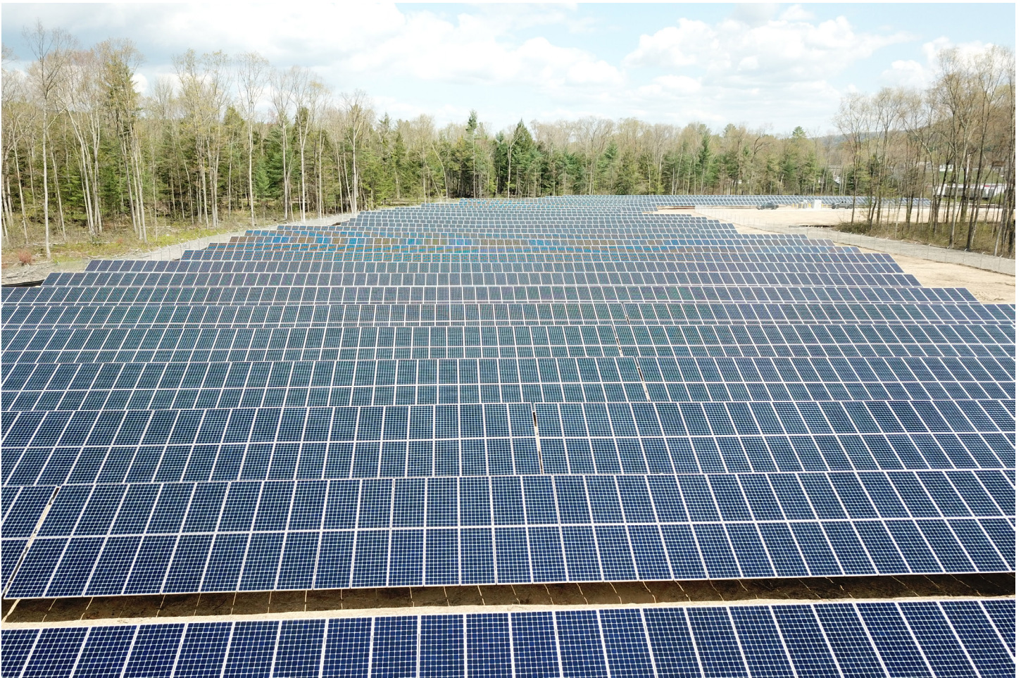
Solar panels installed at Canaan, CT site. A total of 2.9 mega-watts are generated from solar panels at this site.
