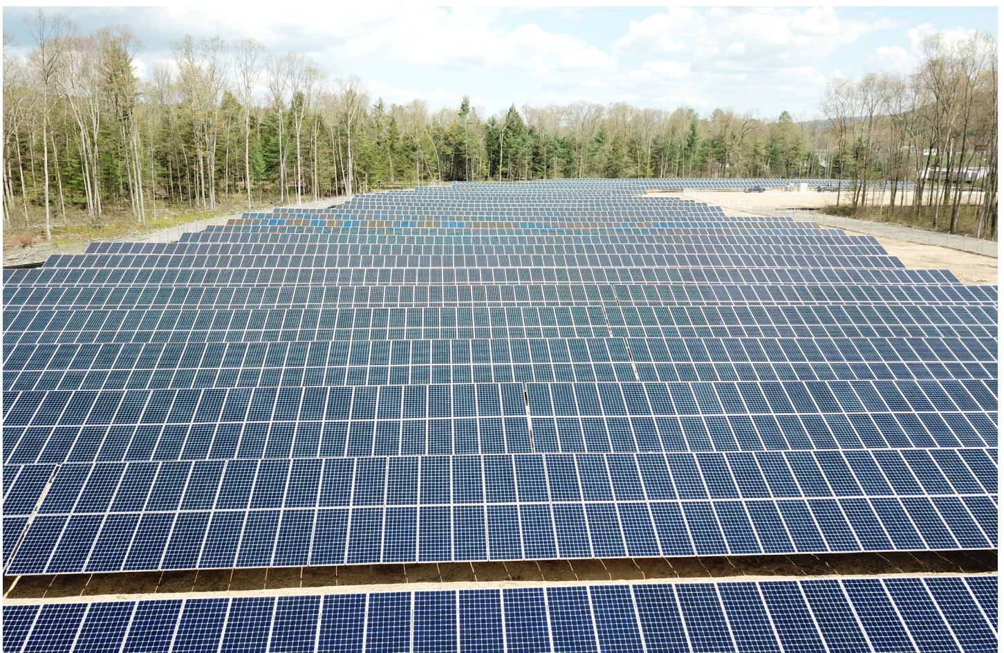
Solar panels installed at Canaan, CT site. A total of 2.9 mega-watts are generated from solar panels at this site.
