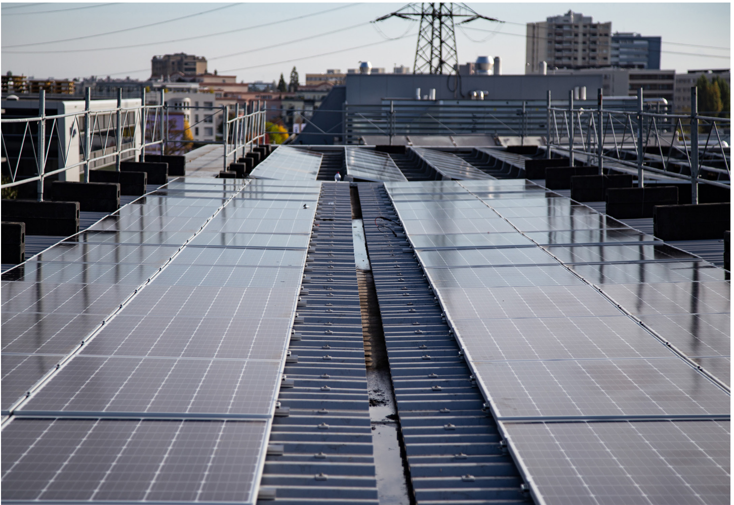
Solar panels installed at the BD European Headquarters in Eysins, Switzerland.
